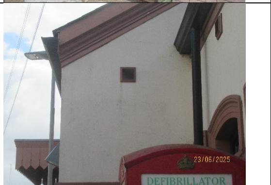
15 – Isambard House wall cracking
